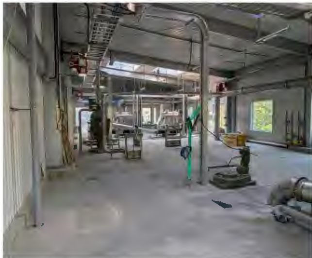
Photo 1: Headworks w/ Grating
