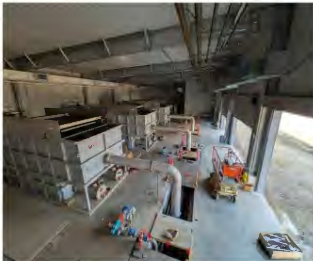
Photo 2: DAF with Sludge Pumps
