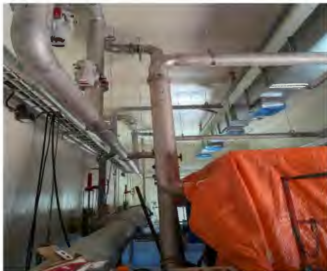
Photo 3: Blower Room Piping
