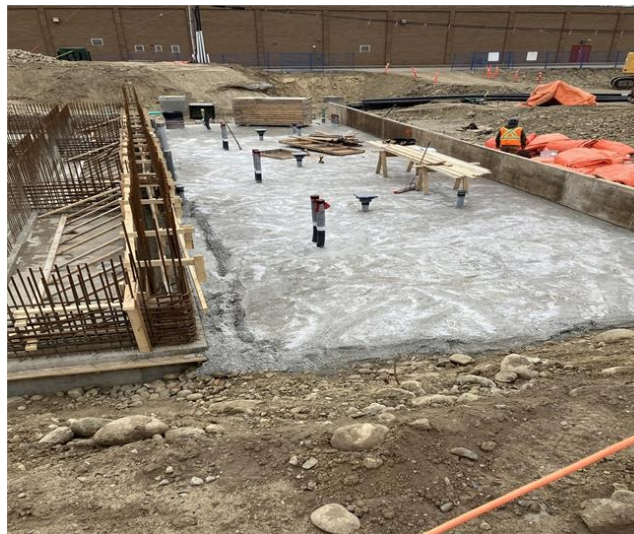
Photo 2: MBBR Blower Room Mudslab
