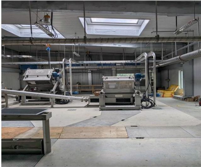
Photo 1: Compactors and screens installed in HW building
