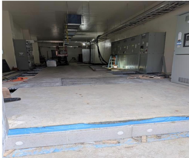
Photo 4: DAF Electrical Main Breaker, Switchgear and MCC 800
